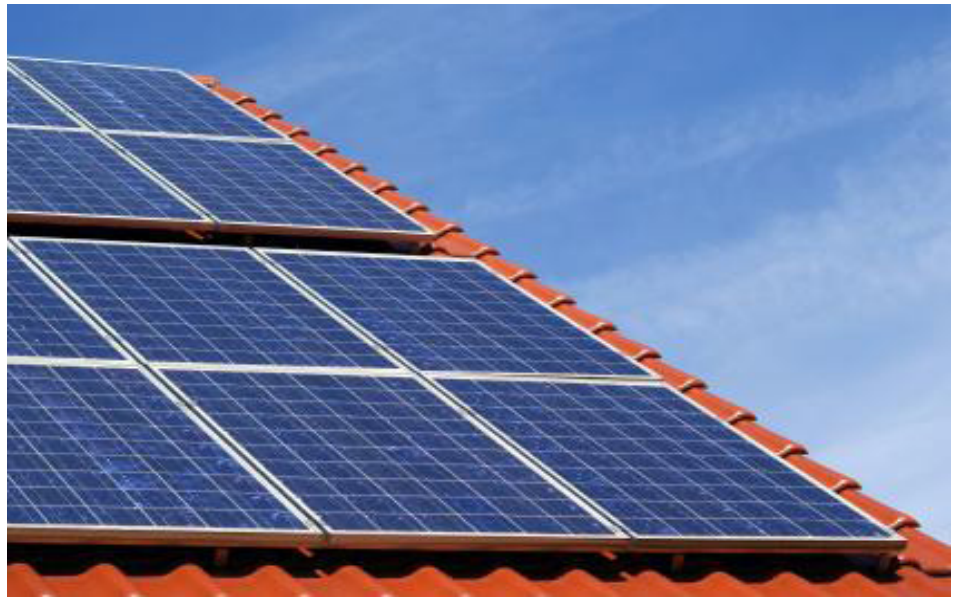
Polycrystalline solar panel
