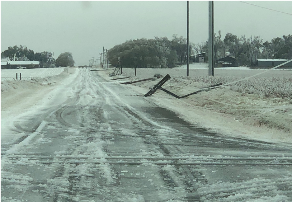
CKenergy power lines buckle under the heavy weight of ice
