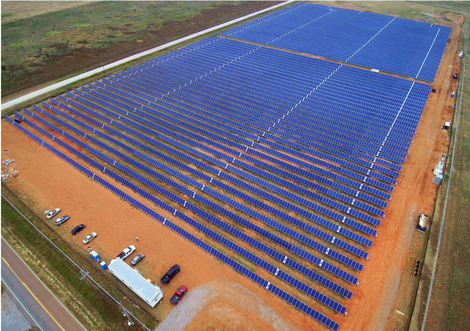
Aerial view of the new solar farm located at the Pine Ridge substation. Photo Courtesy of Western Farmer's Electric Co-op.
